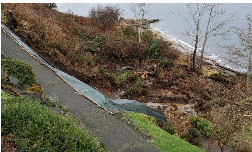
Surficial landslide, Discovery Drive, January 2021 with approximately 90% of the fully saturated slope failing.
